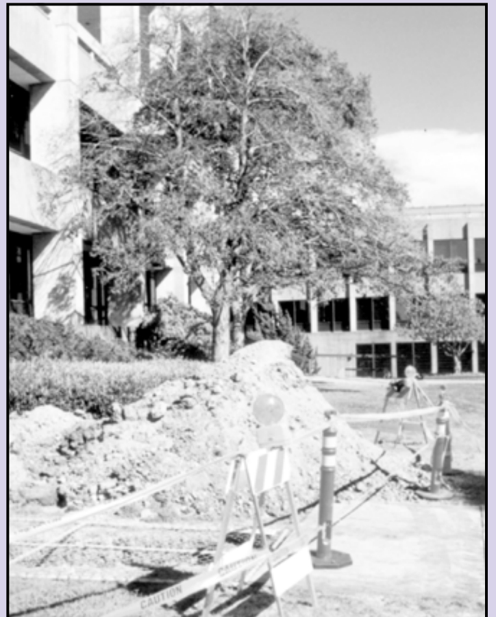
Under Construction: Those heaps of soil around Warren hall indicate work is under way on the campus' multi-million-dollar recabbling project.
